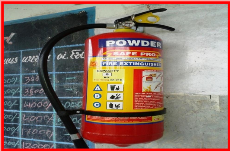
MDM: Fire Extinguisher in working condition.
